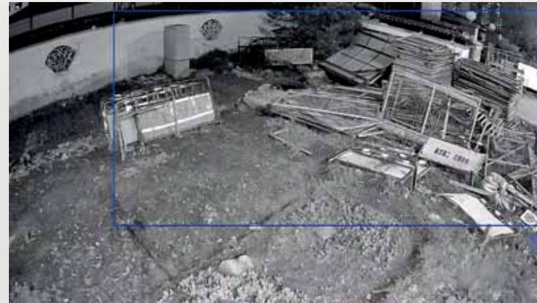
You are in the danger zone, do not approach
